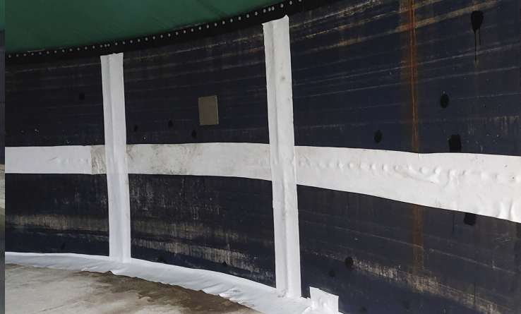
Pic. 2: Secutex® protection strips in the area of the outstanding heads of the screws
