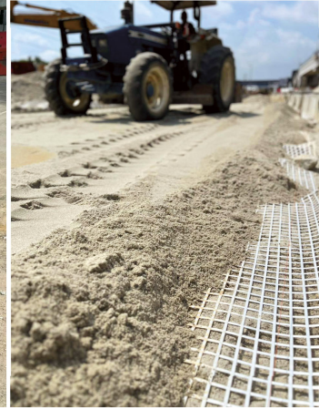
Fig. 2: Road in need of repair (left) and reconstruction with Naue Secugrid® geogrid (right)
