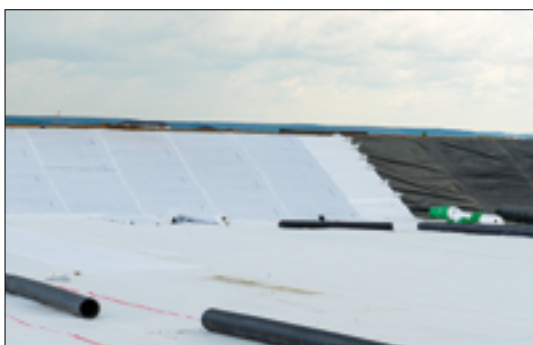
Figure 17: Secudrain® WD drainage system in stormwater retention pond
