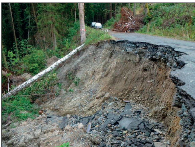
Fig. 3: Road collapse due to erosion damage
