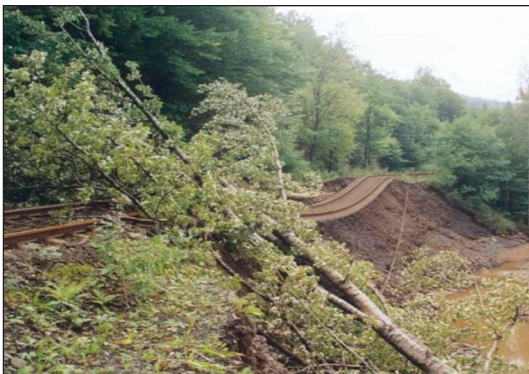
Fig. 2: Undermined rail track
