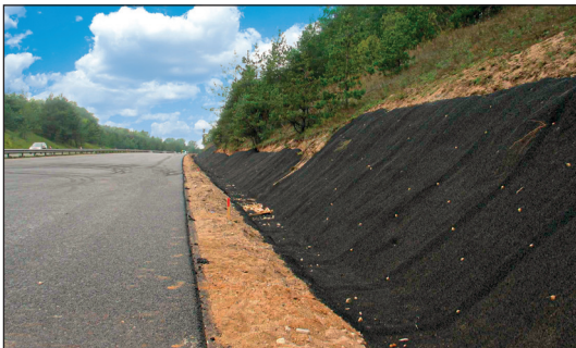
Fig. 3: Embankment with erosion control system
