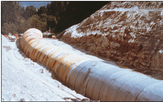
Figure 68 Secudrain® as precipitation and groundwater collector on a tunnel (Pustertal, Italy)
