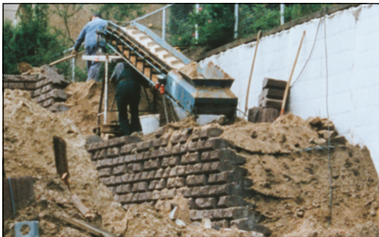
Figure 64 Drainage of a retaining wall with Secudrain®
