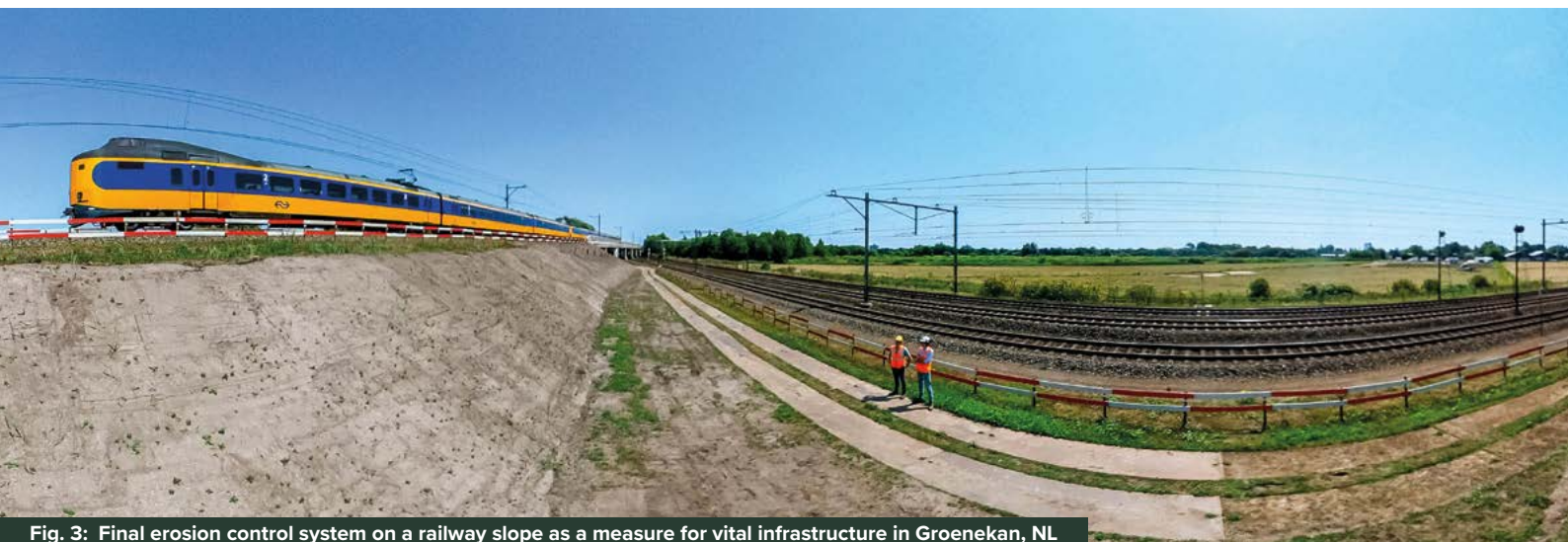
Fig. 3: Final erosion control system on a railway slope as a measure for vital infrastructure in Groenekan, NL
