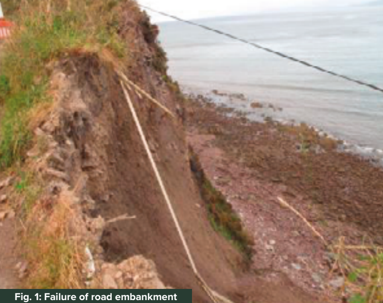
Fig. 1: Failure of road embankment
