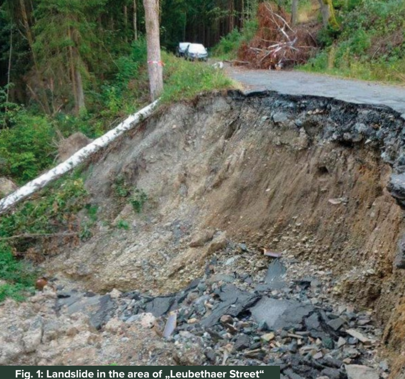
Fig. 1: Landslide in the area of „Leubethaer Street“
