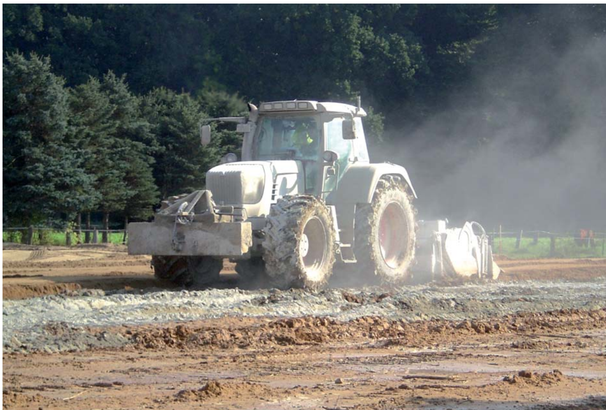
Fig. 7: Example of base soil improvement by milling of binder (lime/cement) into the soil
