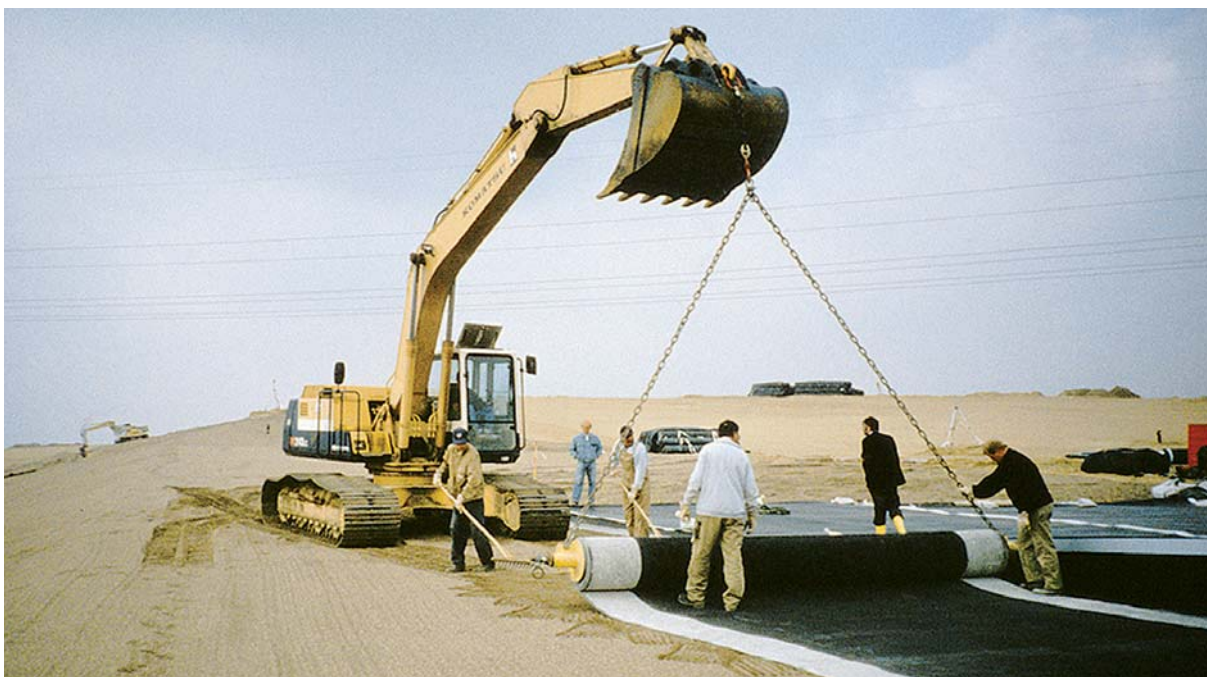
Fig. 2: Installation of the geosynthetic clay liner (GCL) as part of a geosynthetic cover system at the landfill Neu Wulmstorf near Hamburg, Germany, 1996/97
