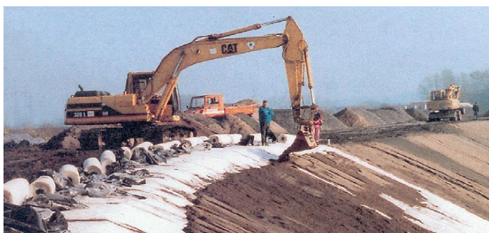
Fig. 4 Lippe River levee reconstruction (1994): Installing Bentofix® GCL as a levee seal (Saathoff & Werth 2003)
