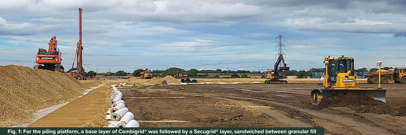
Fig. 1: For the piling platform, a base layer of Combigrid® was followed by a Secugrid® layer, sandwiched between granular fill
