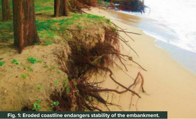
Fig. 1: Eroded coastline endangers stability of the embankment.
