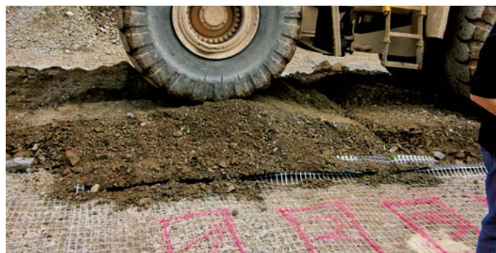
Figure 15: Installation damage factor ( RF_{ID} / A_2 ) determined by a field trial in a quarry
