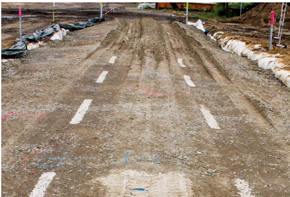
Figure 21: Low rut depth in the Secugrid® geogrid reinforced test section (in the front) compared to the unreinforced test section (in the back)
